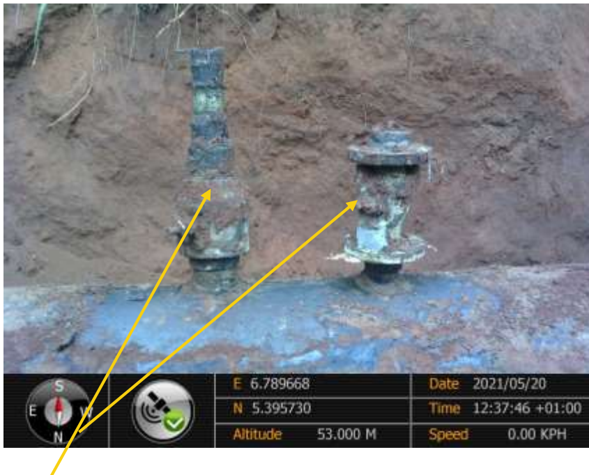
Close-up: 3inch and 2inch ball valves installed at 12 o'clock position on 16inch Egbema Assa Pipeline at Obile. Picture was taken during Joint Investigation of 20 th May 2021.
