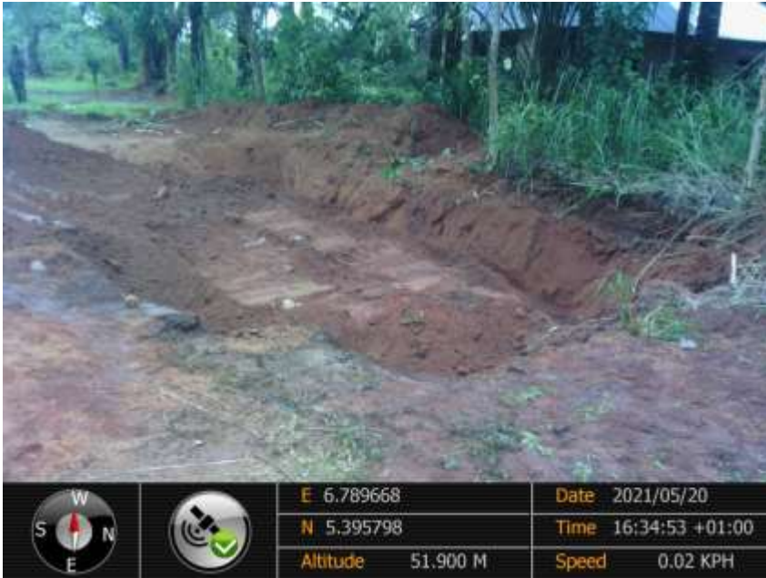
Overview: Part of spill impact on 16inch Egbema Assa Pipeline at Obile. Picture was taken during Joint Investigation of 20 th May 2021.
