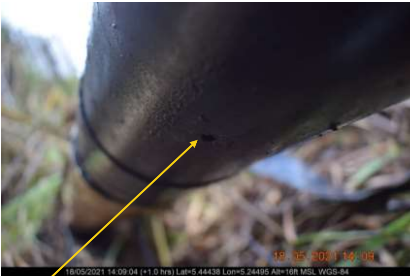
Close-up: Pinhole at 7 o'clock position on 4inch Yokri Well 111T Flowline at Yokri . Picture was taken during Joint Investigation of 18 th May 2021.
