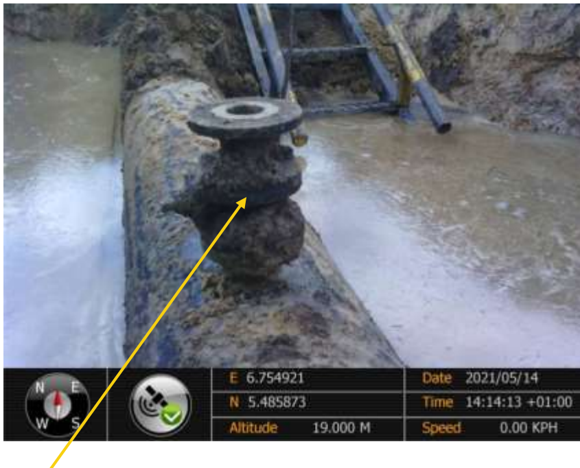
Close-up: 2inch ball valve installed at 12 o'clock position on 16inch Egbema Assa Pipeline at Etekwuru. Picture was taken during Joint Investigation of 14 th May 2021.
