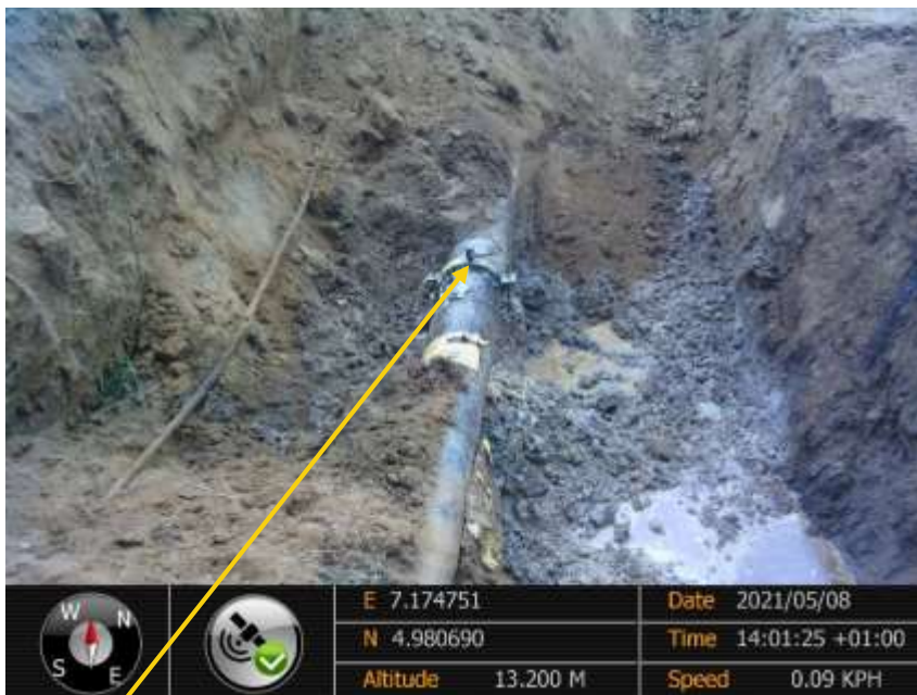
Close-up: Local fabricated clamp fitted with 1 inch ball valve installed at 12 o'clock position on 12inch ImoRiver 2 – Ogale Pipeline at Owaza. Picture was taken during Joint Investigation of 8 th May 2021.
