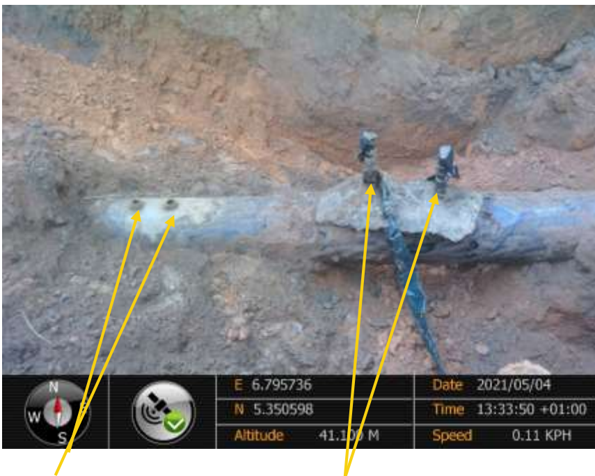
Close-up: 2nos of 2inch non leaking ball valves and 2nos of 2inch leaking ball valves installed at 12 o'clock position on 18inch Assa Rumuekpe Pipeline at Ochia . Picture was taken during Joint Investigation of 4 th May 2021.
