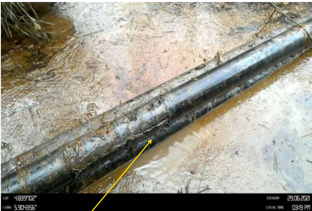
Close-up: Hacksaw cut at 3 o'clock position on 6inch Seibou Bulkline at Tububou. Picture was taken during Joint Investigation of 29 th June 2021.
