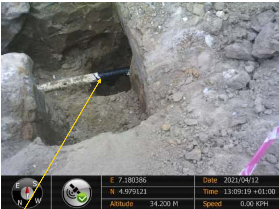
Close-up: Pinhole at 7 o'clock position on 3inch Imo River Well 63T Flowline at Owaza. Picture was taken during Joint Investigation of 12 th April 2021.
