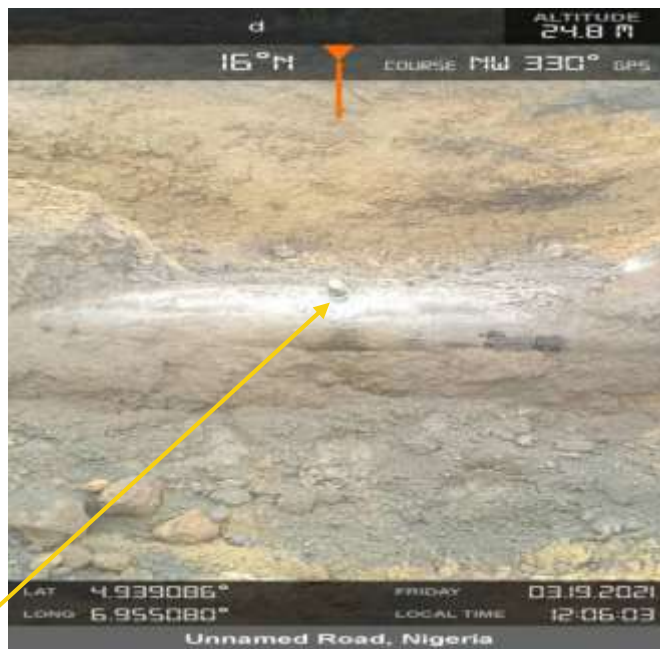
Close-up: 2inch illegal connection installed at 12 o'clock on 20inch Rumuekpe Nkpoku Trunkline at Mbodo Aluu. Picture was taken during Joint Investigation of 19 th March 2021.
