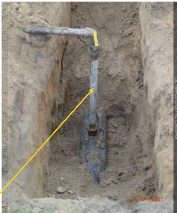
Close-up: 1.5inch crude oil theft valve installed at 12 o'clock position on 8inch Afam Well 27T Flowline at Egberu Picture was taken during Joint Investigation of 2nd April 2021 .
