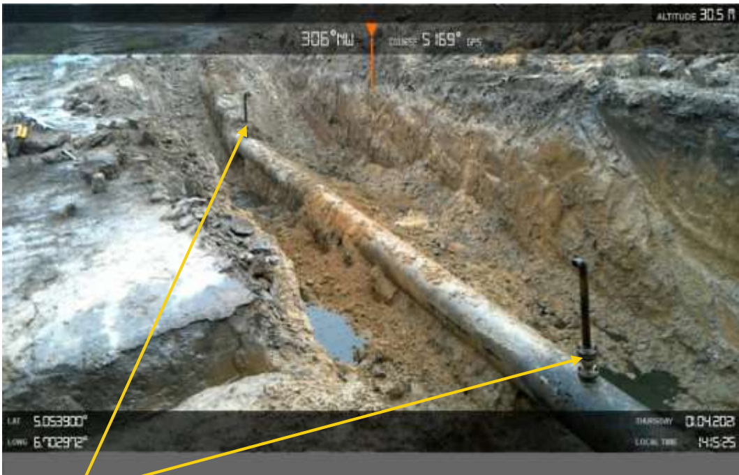
Close-up: 2 nos of crude oil theft installed at 12 o'clock position on 18inch Assa - Rumuekpe Pipeline at Elele Alimini. Picture was taken during Joint Investigation of 1 st April 2021.
