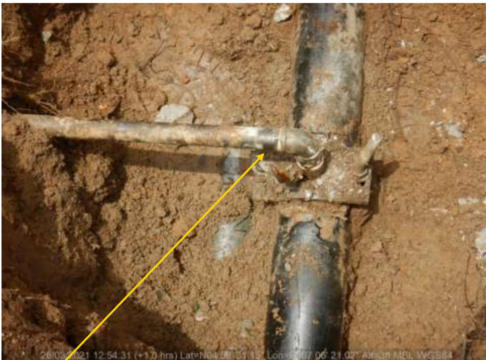
Close-up: SP 1 : Crude oil theft point installed at 12 o'clock position on 4inch Nkali well 10S flowline at Odagwa . Picture was taken during Joint Investigation of 26 th March 2021.
