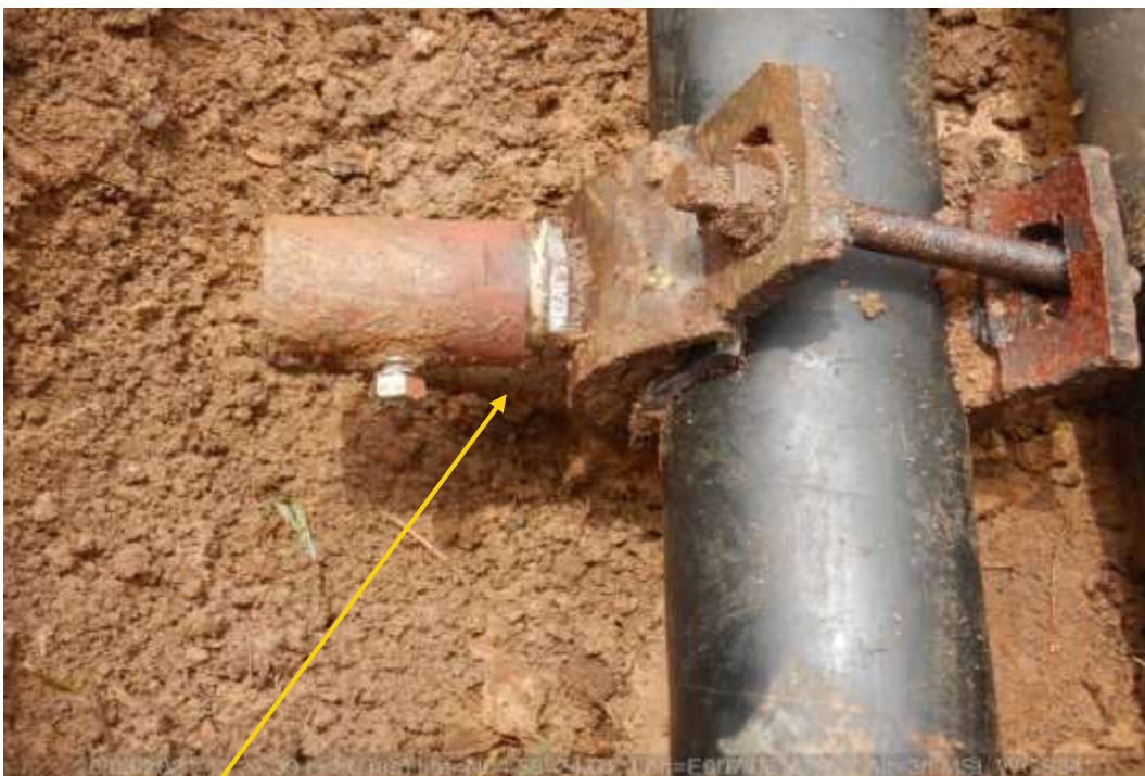
Close-up: SP 1 : Crude oil theft points installed at 3 and 9 o'clock position on 4inch Nkali well 13L/S flowline at Odagwa 2. Picture was taken during Joint Investigation of 26 th March 2021.
