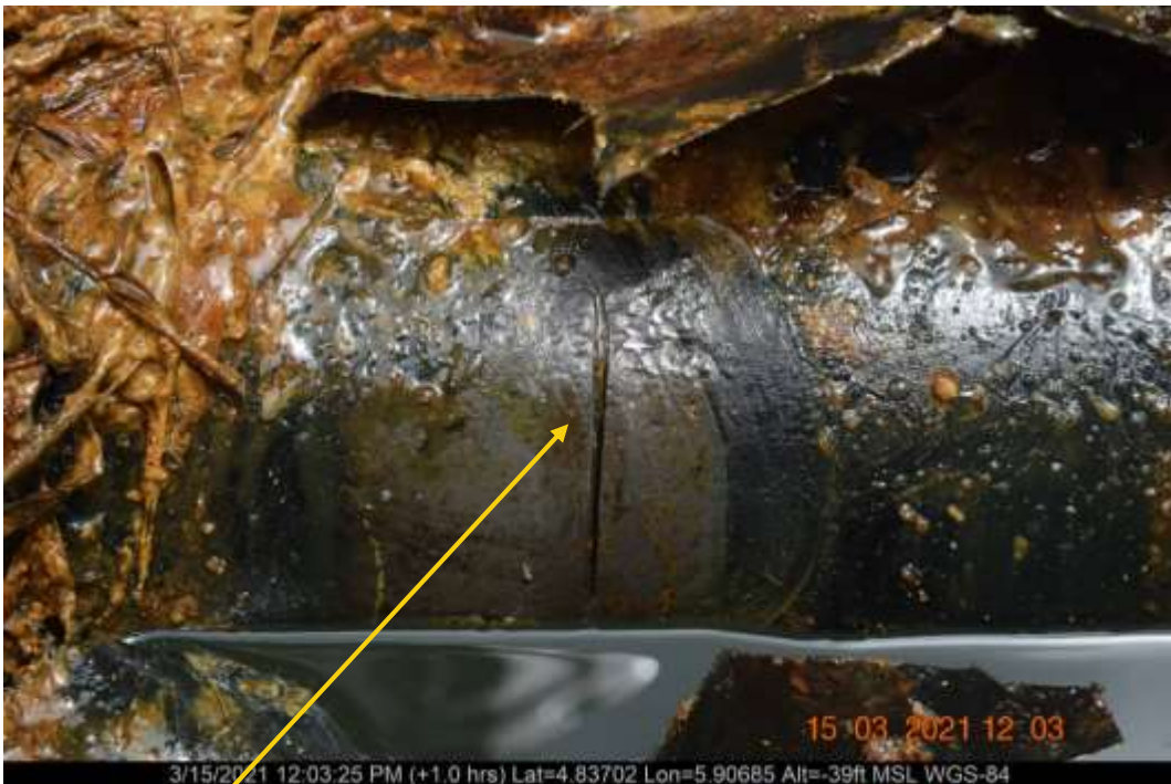
Close-up: SP 1 : 2nos hacksaw cut at 3 and 9 o'clock position on 6inch Seibuo Well 3 and 4 bulkline at Ogbeinbiri. Picture was taken during Joint Investigation of 15 th March 2021.
