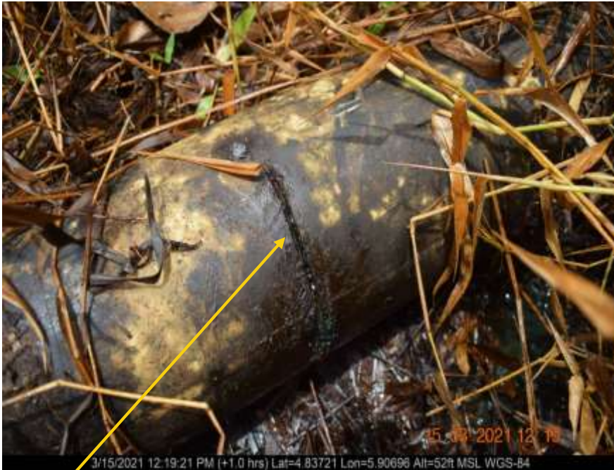
Closeup : SP 2: : 2nos hacksaw cut at 3 and 9 o'clock position on 6inch Seibuo Well 3 and 4 bulkline at Ogbeinbiri. Picture was taken during Joint Investigation of 15 th March 2021.
