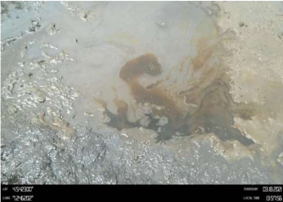
Overview: Part of spill impact on 28inch Bomu Bonny Pipeline at Owokiri. Picture was taken during Joint Investigation of 18 th March 2021.
