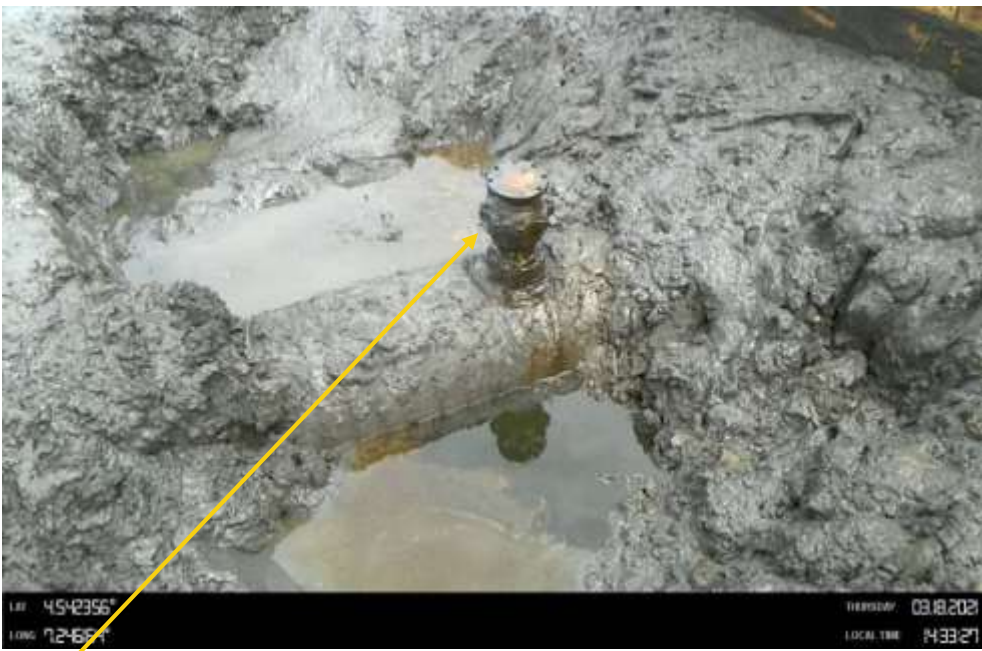
Close-up: Crude oil theft point installed at 12 o'clock position on 28inch Bomu Bonny Pipeline at Owokiri. Picture was taken during Joint Investigation of 18 th March 2021.
