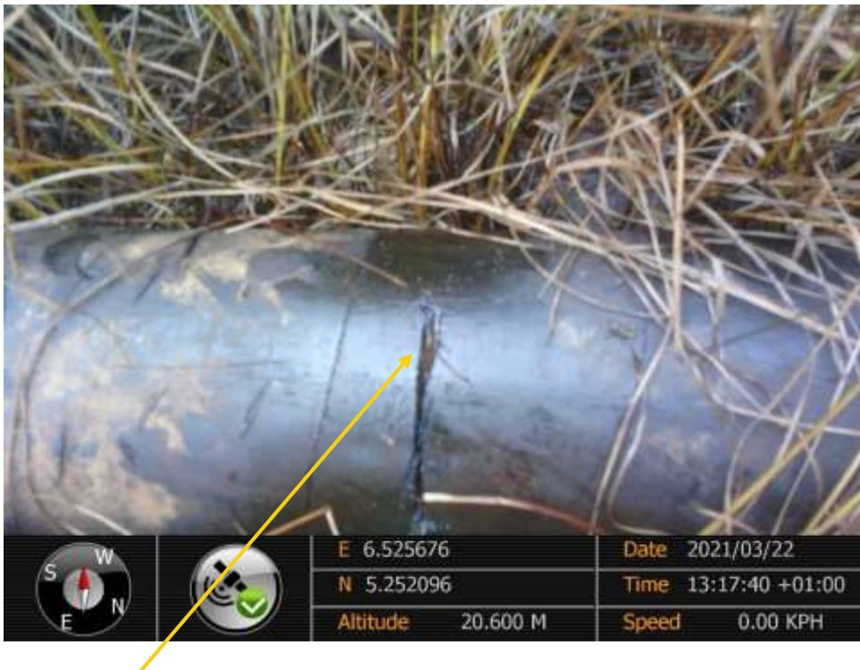
Close-up: SP 1: Hacksaw cut from 10-12 o'clock position on 4inch (Bulkline) well 4 Flowline at Biseni. Picture was taken during Joint Investigation of 22 nd March 2021.
