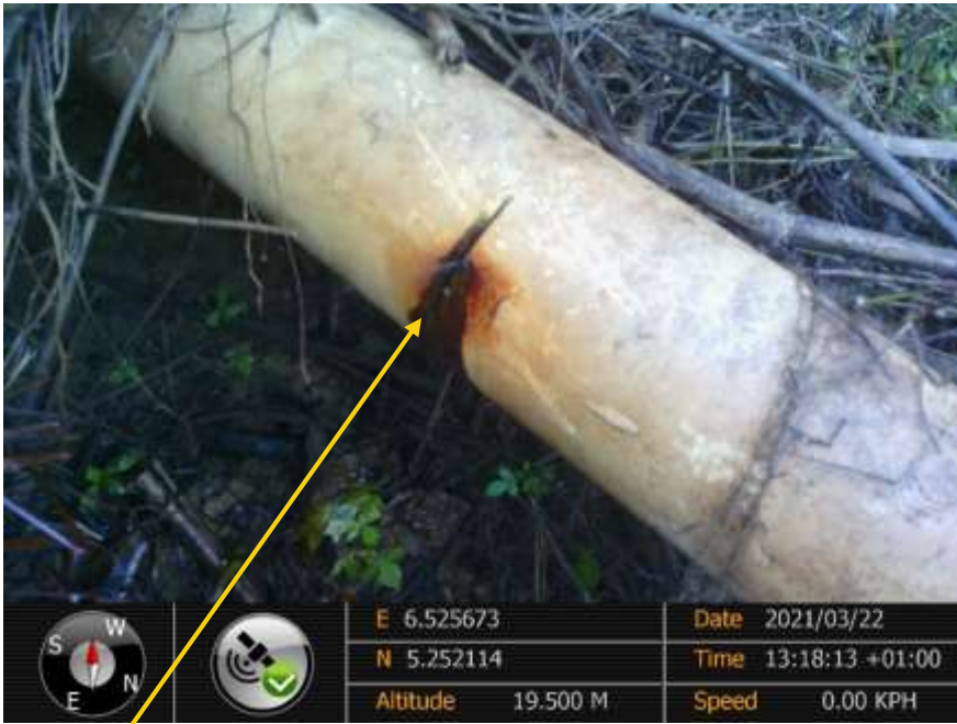
Closeup: SP 2 Hacksaw cut from 9-11 o'clock position on 4inch (Bulkline) well 4 Flowline at Biseni. Picture was taken during Joint Investigation of 22 nd March 2021.
