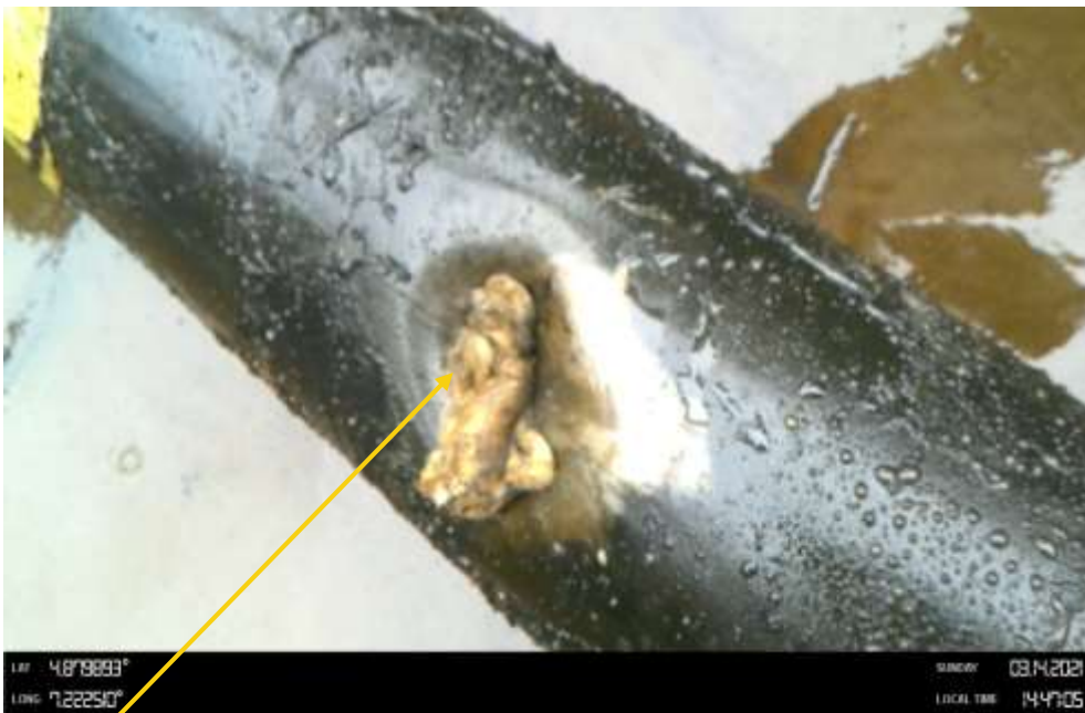
Close-up: Plugged inward dent and sharp edge hole between 10 to 12 o'clock position on 8inch Isimiri Imo gate Pipeline at Umuelechi. Picture was taken during Joint Investigation of 14 th March 2021.
