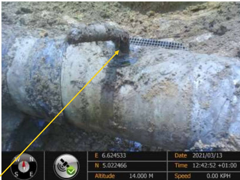
Close-up: 2inch nipple installed at 12 o'clock position on 14inch Okordia Rumuekpe Pipeline at Edeoha. Picture was taken during Joint Investigation of 13 th March 2021.
