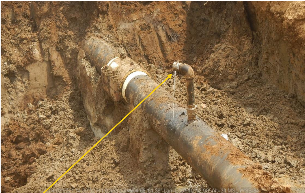
Close-up: Crude oil theft point installed at 12 o'clock position on 12inch Imo River2 – Imo River1 Pipeline at Odagwa. Picture was taken during Joint Investigation of 4 th March 2021.
