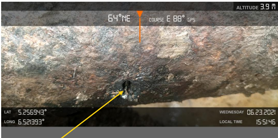
Closeup 2: Two of three nos spill points puncture on Adibawa North East Well 1 Flowline at Biseni. Picture was taken during Joint Investigation of 23 rd June 2021.
