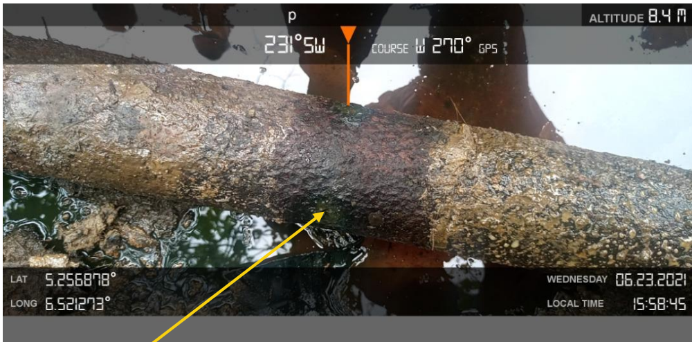
Closeup 3: Three of Three nos spill points puncture on Adibawa North East Well 1 Flowline at Biseni. Picture was taken during Joint Investigation of 23 rd June 2021.
