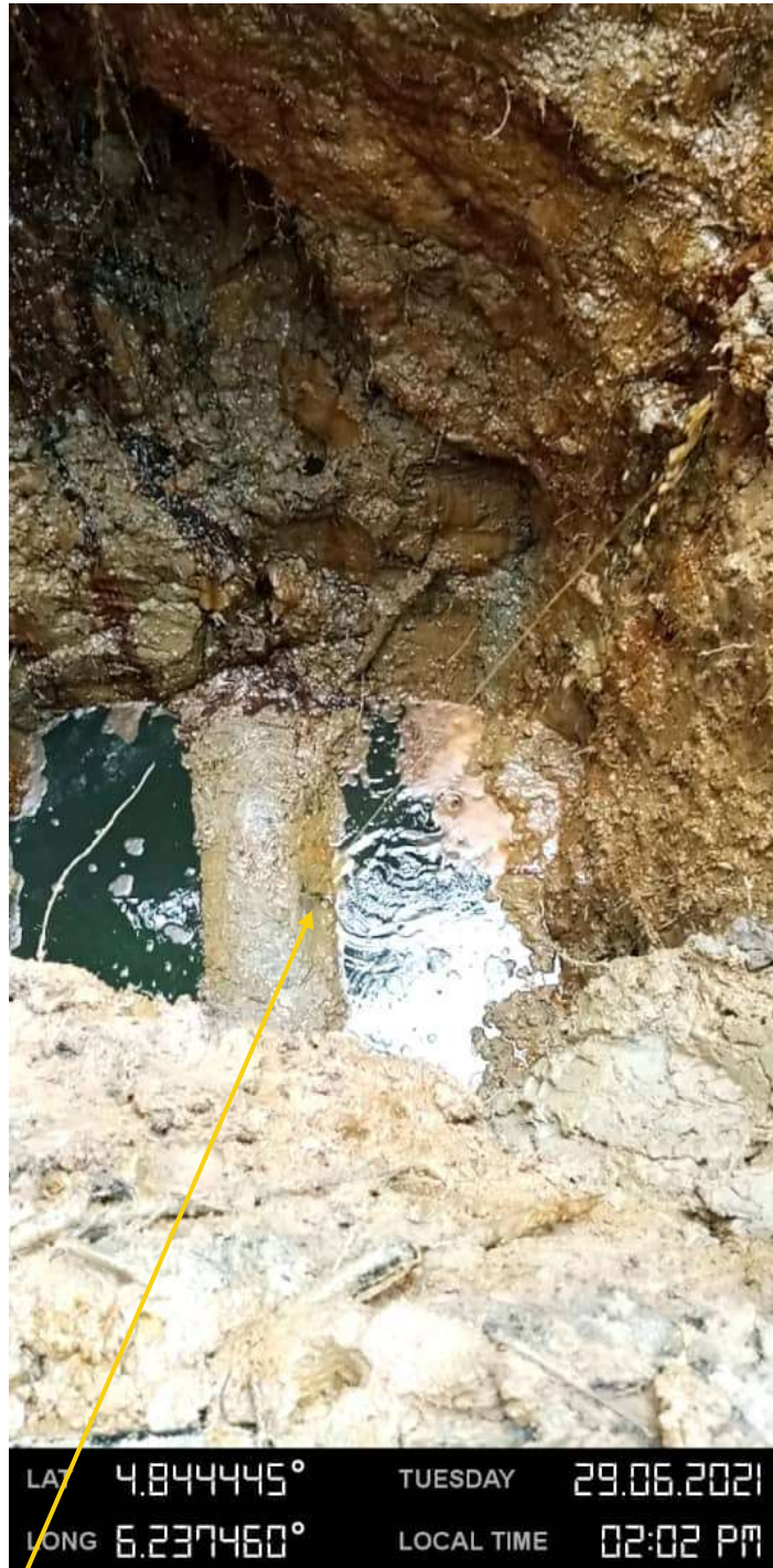
Close-up : Hacksaw cut (2cm length) at 1 o'clock position on 16inch Nun-River to Kolocreek Pipeline at Otuegwe Picture was taken during Joint Investigation of 29 th June 2021.
