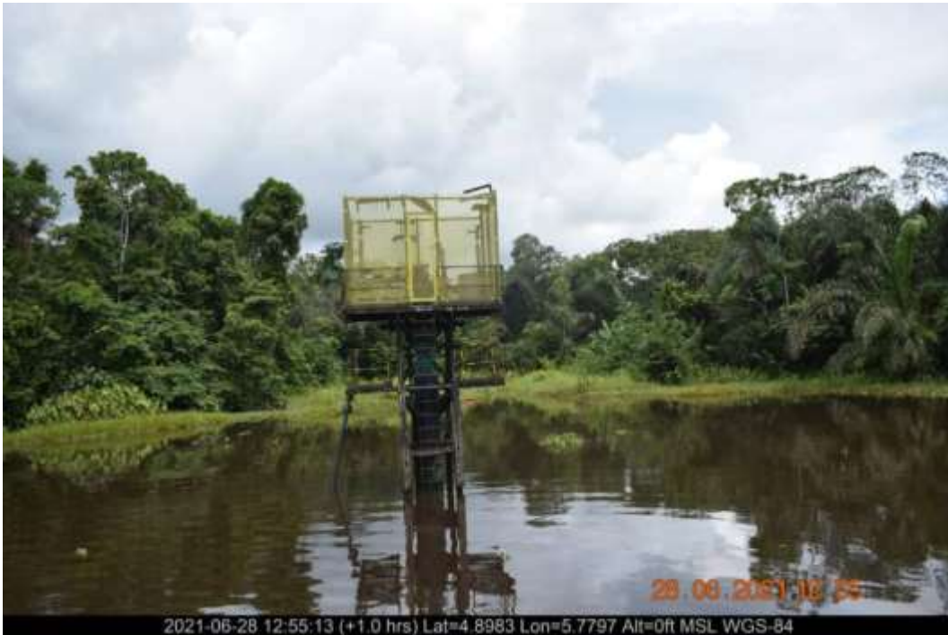
Overview: Part of spill impact on 3inch Opukushi Well 12 L/S Flowline at Agbidiana. Picture was taken during Joint Investigation of 28 th June 2021.
