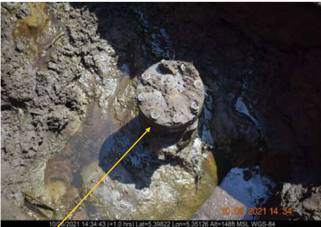
Close-up: Weld on 4inch valve installed at 12 o'clock position on 24inch Trans Escravos Pipeline at Obotobo. Picture was taken during Joint Investigation of 10 th June 2021.
