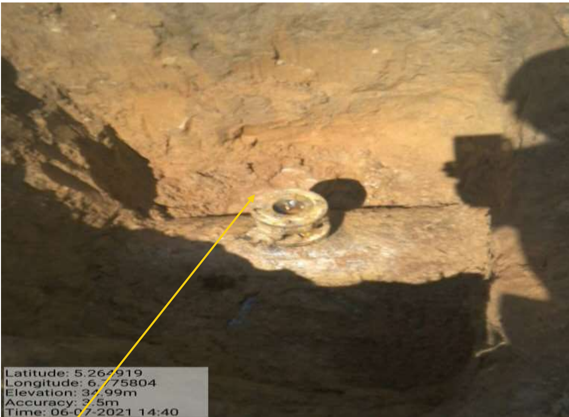
Close-up: 2inch ball valve installed at 12 o'clock position on 18inch Egbema Assa Pipeline at Egbeda. Picture was taken during Joint Investigation of 7 th June 2021.
