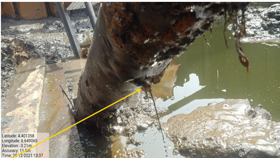
Close-up: 20mm Rough-edge Hole due to corrosion at 6 o'clock position on 6'' Belema Delivery line at Belema. . Picture was taken during Joint Investigation of 20 th December 2021.
