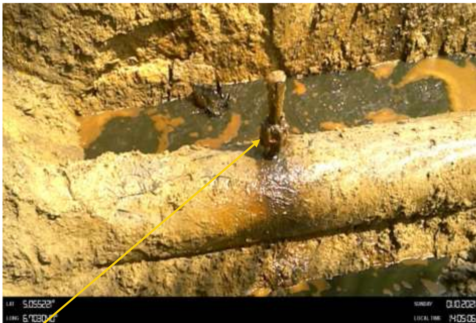
Close-up: Plugged crude oil theft point installed at 12 o'clock position on 18inch Assa Rumuekpe Pipeline at Elele-Alimini. Picture was taken during Joint Investigation of 10 th January 2021.
