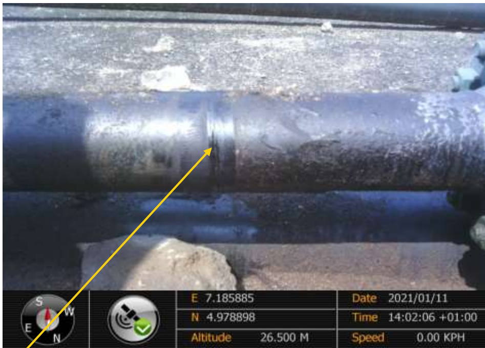
Close-up: Hacksaw cut from 7o'clock to 11o'clock position on 4inch Imo River well 22s Flowline at Owaza. Picture was taken during Joint Investigation of 11 th January 2021.
