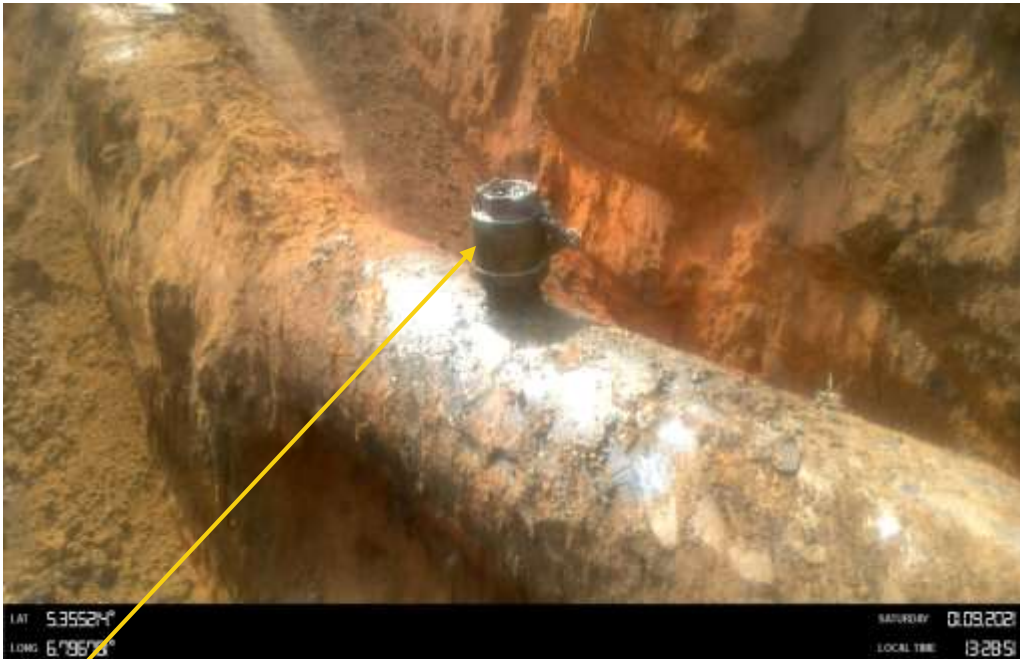
Close-up: 3inch ball valve installed at 12 o'clock position on 18inch Assa Rumuekpe Pipeline at Ububo Ochia. Picture was taken during Joint Investigation of 9 th January 2021.
