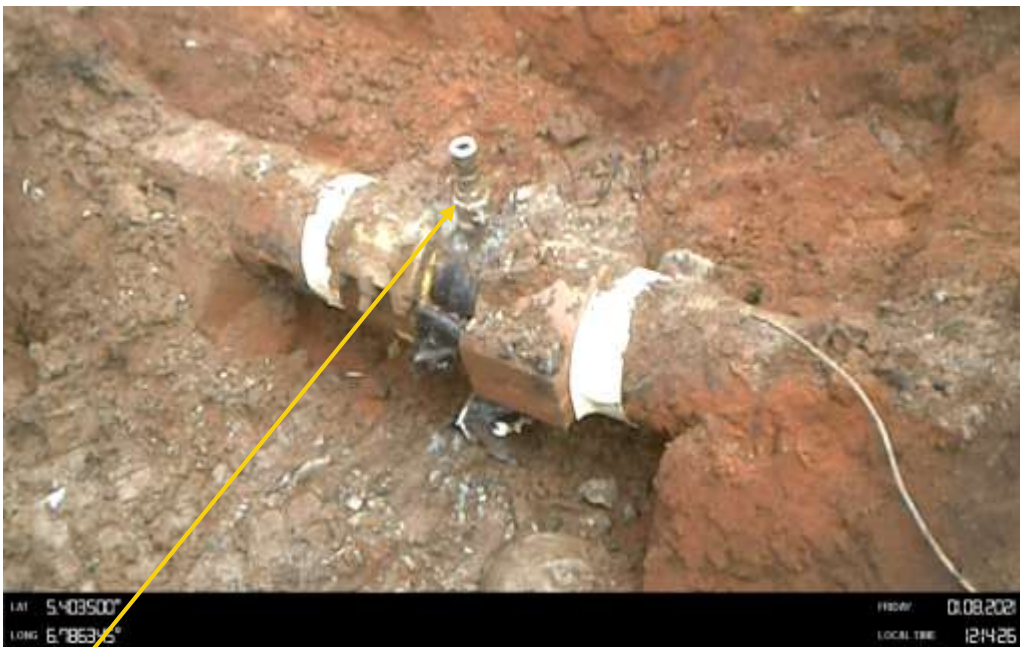
Close-up: 2.5inch ball valve with 2inch pipe connection installed at 12 o'clock position on 16inch Egbema Assa Pipeline at Obile. Picture was taken during Joint Investigation of 8 th January 2021.
