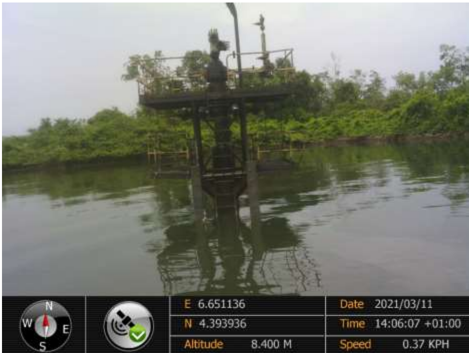
Overview: Part of spill impact on Belema well 8 Wellhead at Belema. Picture was taken during Joint Investigation of 11 th March 2021.
