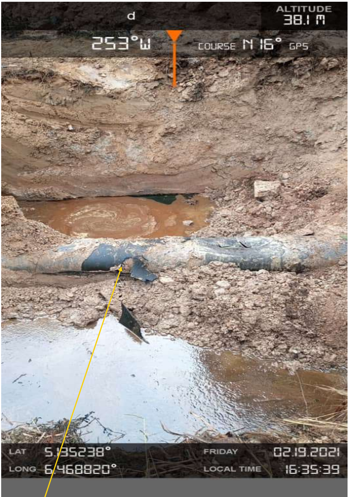
Close-up 1: A Tear at Point 1 ( 6 o'clock position) on 14inch Okordia Rumuekpe Pipeline at Ikarama . Picture was taken during Joint Investigation of 19 th Feb 2021.
