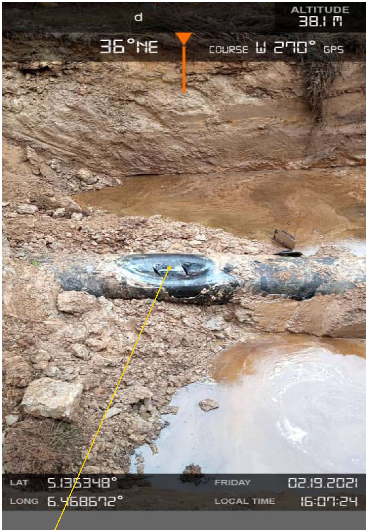
Close-up 2: Inward dent/double cut at point 2 ( 12 o'clock position) on 14inch Okordia Rumuekpe Pipeline at Ikarama . Picture was taken during Joint Investigation of 19 th Feb 2021 .
