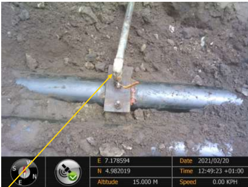
Close-up: 1.5inch Crude oil theft valve installed at 12 o'clock position on 6inch Imo River Well 26s Flowline at Owaza. Picture was taken during Joint Investigation of 20 th February 2021.
