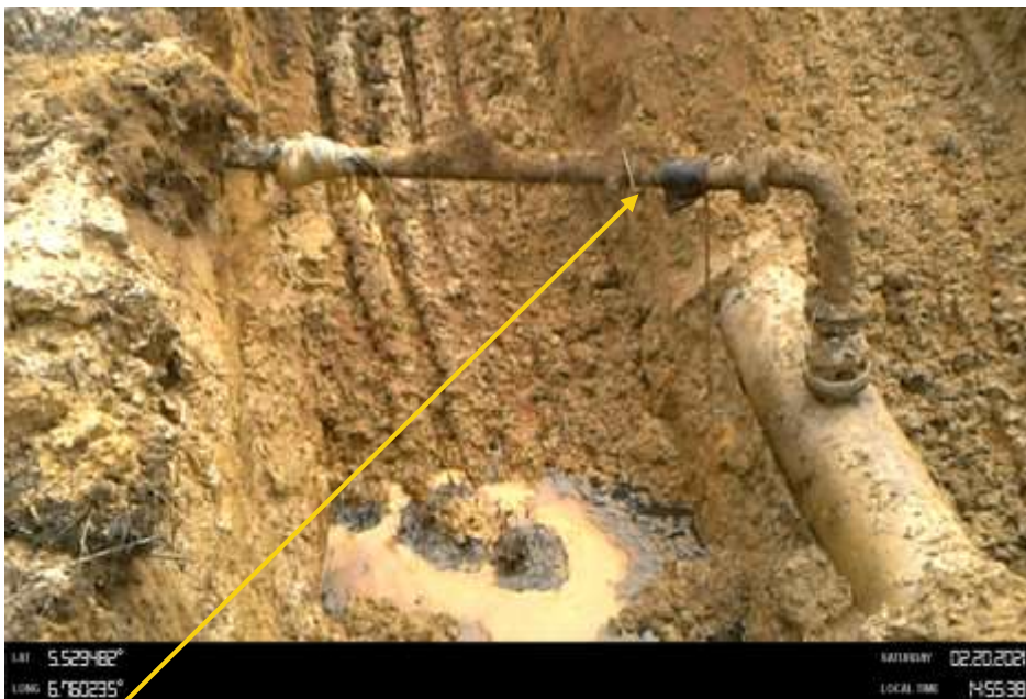
Close-up: Crude oil theft point installed at 12 o'clock position on 16inch Assa Egbema Pipeline at Obiakpu . Picture was taken during Joint Investigation of 20 th February 2021.
