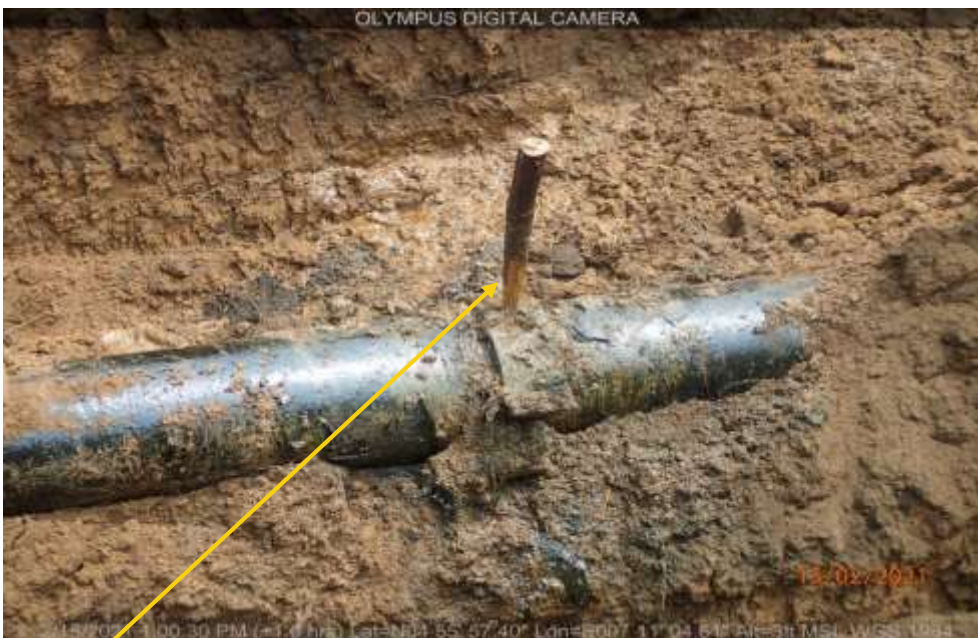
Close-up: Plugged 2inch Crude oil theft point installed at 12 o'clock position on 12inch Imo River Ogale Pipeline . Picture was taken during Joint Investigation of 15 th February 2021.
