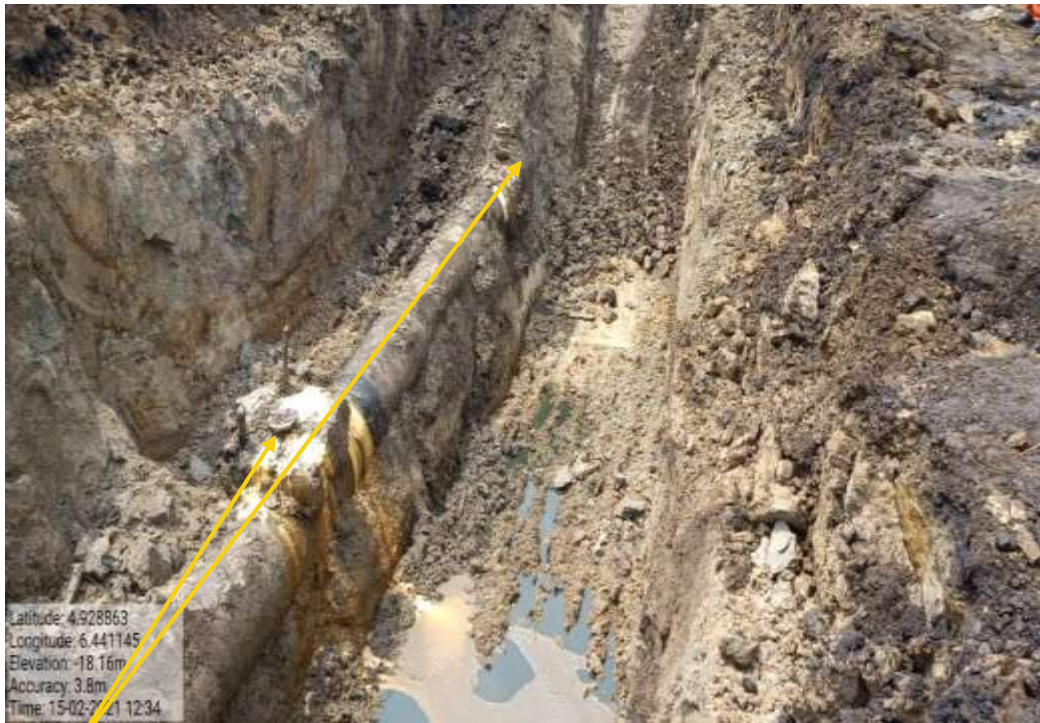
Close-up: 4inch valve with a concrete cast and a non-leaking 4inch valve of 5.2m apart installed at 12 o'clock position on 20inch Kolocreek – Rumuekpe Pipeline at Odau Km9 . Picture was taken during Joint Investigation of 15 th February 2021.
