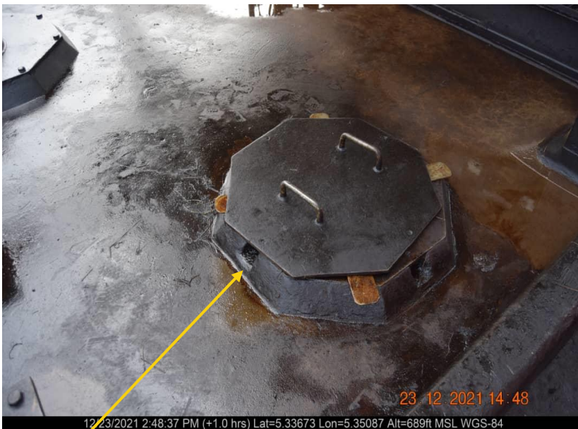
Close-up: Failed Skimming Pit on Forcados Terminal Skimming Pit at Ogulagha. Picture was taken during Joint Investigation of 23 rd December 2021.
