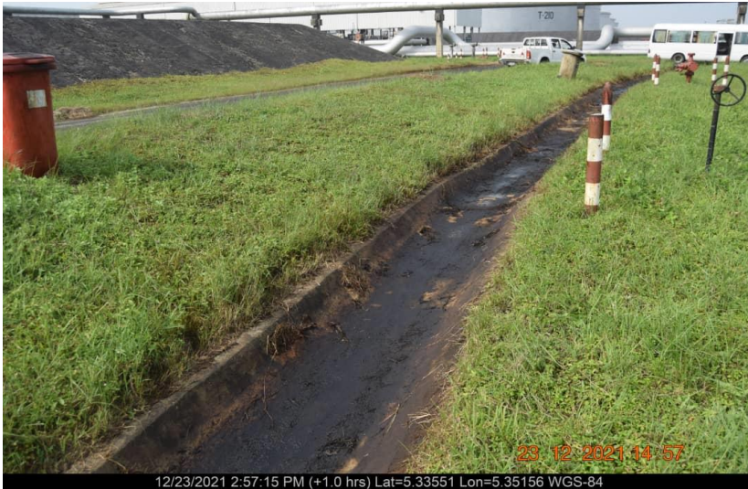
Overview: Part of spill impact on Forcados Terminal Skimming Pit at Ogulagha. Picture was taken during Joint Investigation of 23 rd December 2021.
