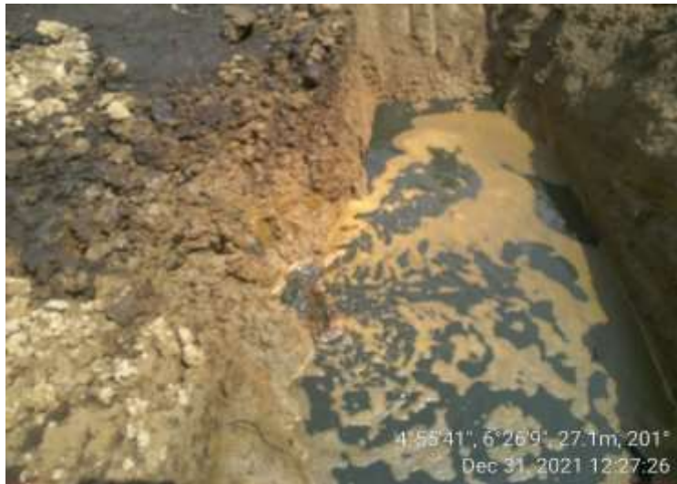
Overview: Part of spill impact on 20" Kolocreek-Rumuekpe Pipeline at Odau. Picture was taken during Joint Investigation of 31 st December 2021.
