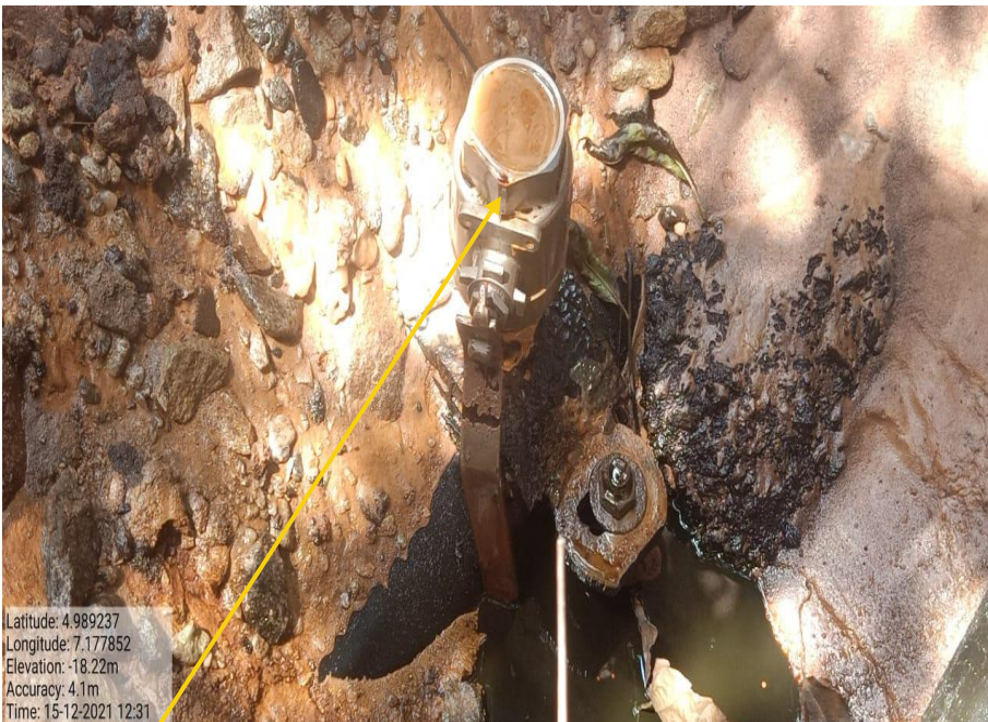
Close-up: 2" Ball valve attached to a local fabricated clamp installed at 12 o'clock position on 4" Imo River Well 64L Flowline at Igiriukwu-Owaza. Picture was taken during Joint Investigation on 15th December 2021.
