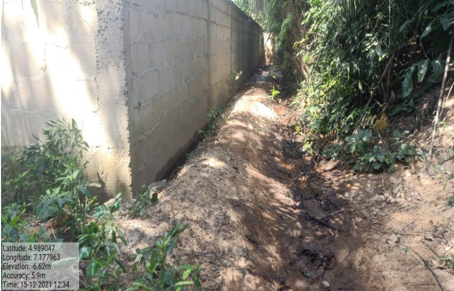
Overview: Part of spill impact on 4" Imo River Well 64L Flowline at Igiriukwu-Owaza. Picture was taken during Joint Investigation on 15th December 2021.
