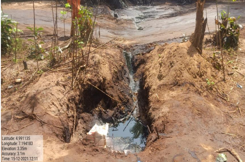
Overview: Part of spill impact on 6" Imo River Well 59T Flowline at Igiriukwu-Owaza. Picture was taken during Joint Investigation on 15th December 2021.
