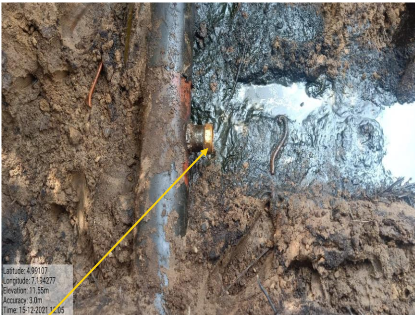
Close-up: 2" Nipple installed at 3 o'clock position on 6" Imo River Well 59T Flowline at Igiriukwu-Owaza. Picture was taken during Joint Investigation on 15th December 2021.
