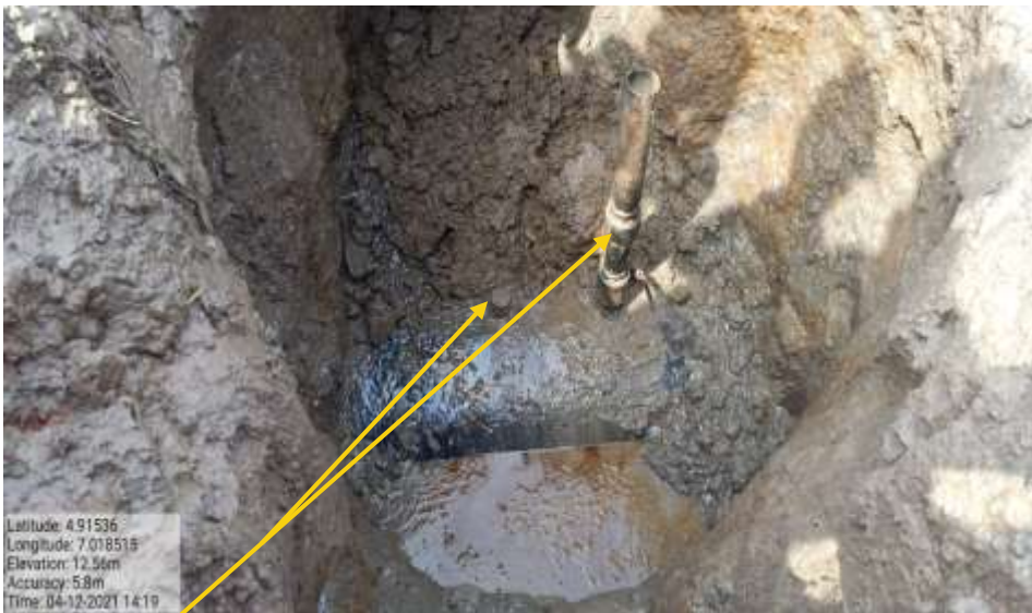
Close-up: 2inch ball valve and 2inch nipple with a distance of 0.2m apart installed at 12 o'clock position on 36" Bomu Bonny Pipeline at Eneka. Picture was taken during Joint Investigation of 4 th December 2021.
