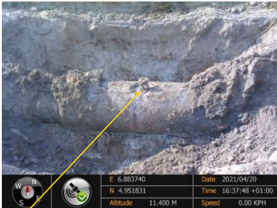
Close-up: 4inch ball valve installed at 12 o'clock position on 36inch Rumuekpe Nkpoku Pipeline at Adanta-lsiokpo . Picture was taken during Joint Investigation of 20 th April 2021 .
