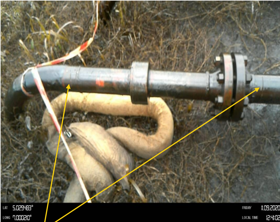
Close-up: Hacksaw cuts of 1.2m apart all at 11 o'clock position on Otamiri Well 7S Flowline at Umuechem. Picture was taken during Joint Investigation on 11th September 2020.
