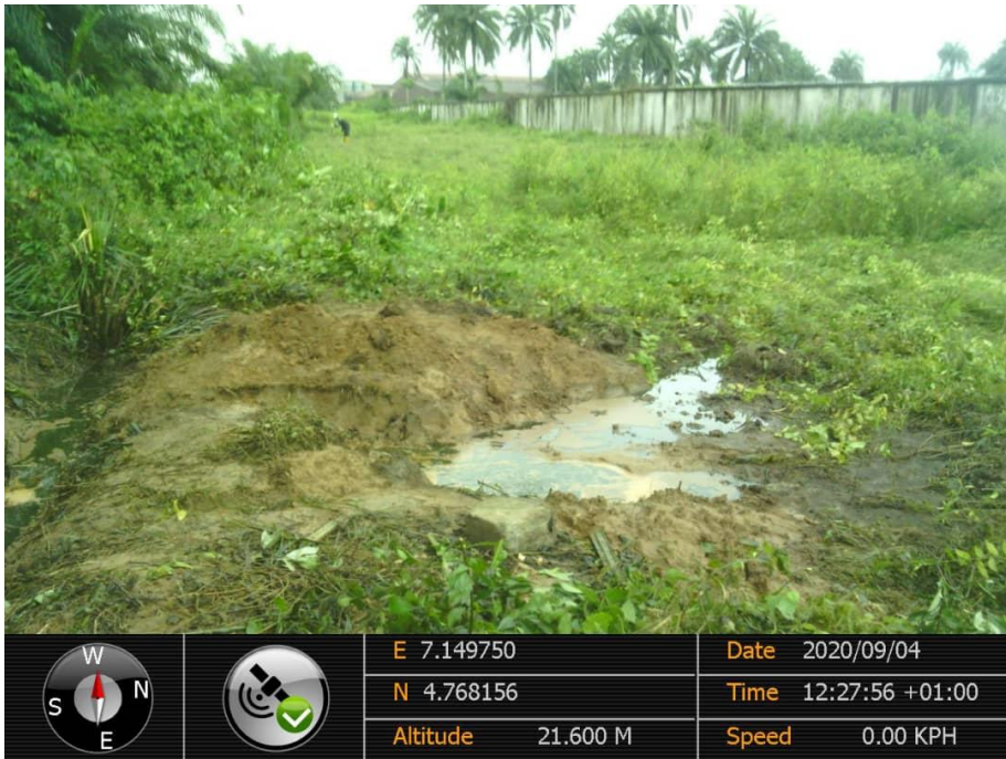
Overview: Part of spill impact on 28" Nkpoku - Bomu Pipeline at Ejamah. Picture was taken during Joint Investigation on 4th September 2020.
