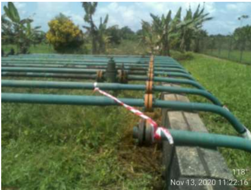
Overview: Part of spill impact on 3inch Nun River Well 11 Lima Flowline at Oporoma. Picture was taken during Joint Investigation on 13th November 2020.
