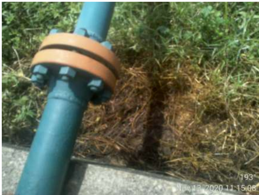
Close-up: Rough edge hole ( Hidding behind the flange) at 6 o'clock position on 3inch Nun River Well 11 Lima Flowline at Oporoma. Picture was taken during Joint Investigation on 13th November 2020.
