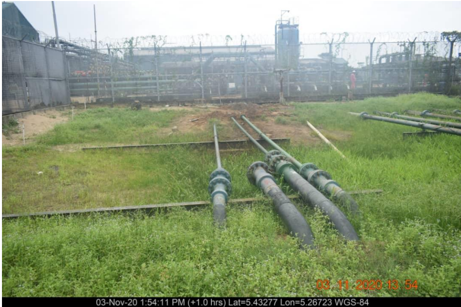
Overview: Part of spill impact on 4" Yokri Well 27 T Flowline at Yokri . Picture was taken during Joint Investigation on 3rd November 2020.
