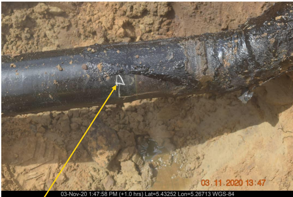
Close-up: Pin hole at 7 o'clock position on 4" Yokri Well 27 T Flowline at Yokri . Picture was taken during Joint Investigation on 3rd November 2020.
