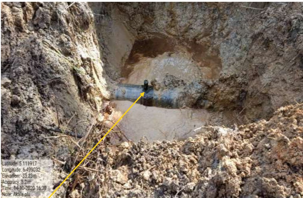
Close-up: Leak point 1. A 2inch threaded ball valve of 98meters apart at 12 o'clock position A section of on 14inch Okordia Rumuekpe Pipeline at Akala-Olu . Picture was taken during Joint Investigation on 14th October 2020.
