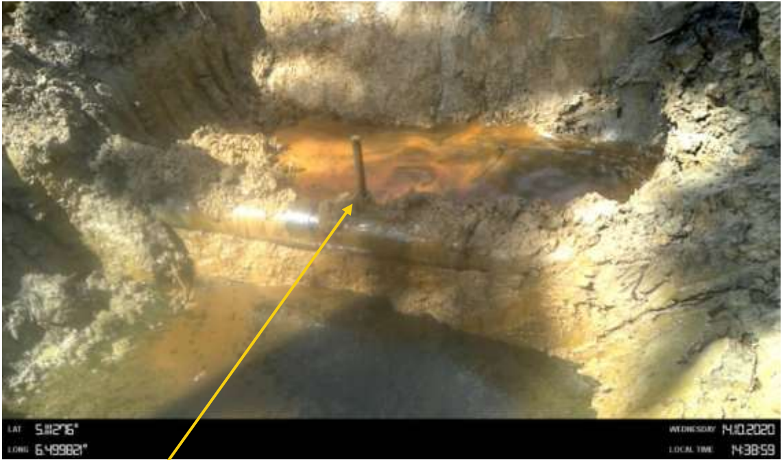
Close-up: Leak point 2 . A 3inch threaded ball valve of 98meters apart at 12 o'clock position A section of on 14inch Okordia Rumuekpe Pipeline at Akala-Olu . Picture was taken during Joint Investigation on 14th October 2020.
