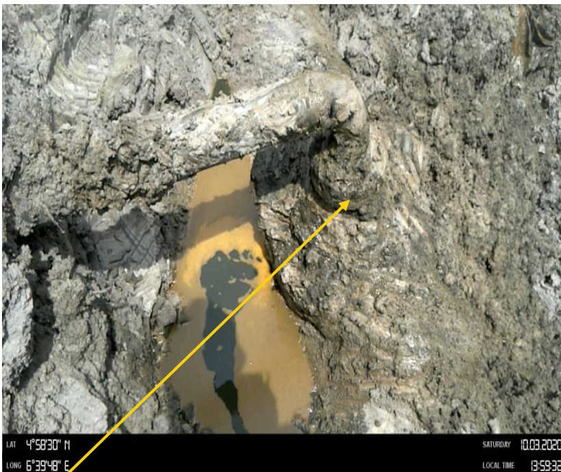
Close-up: 3'' illegal valve with a concrete cast attached to a 3'' galvanized pipe at 12 o'clock position on 20'' Kolocreek –Rumuekpe Pipeline at Ihuowo. Picture was taken during Joint Investigation on 3rd October 2020.
