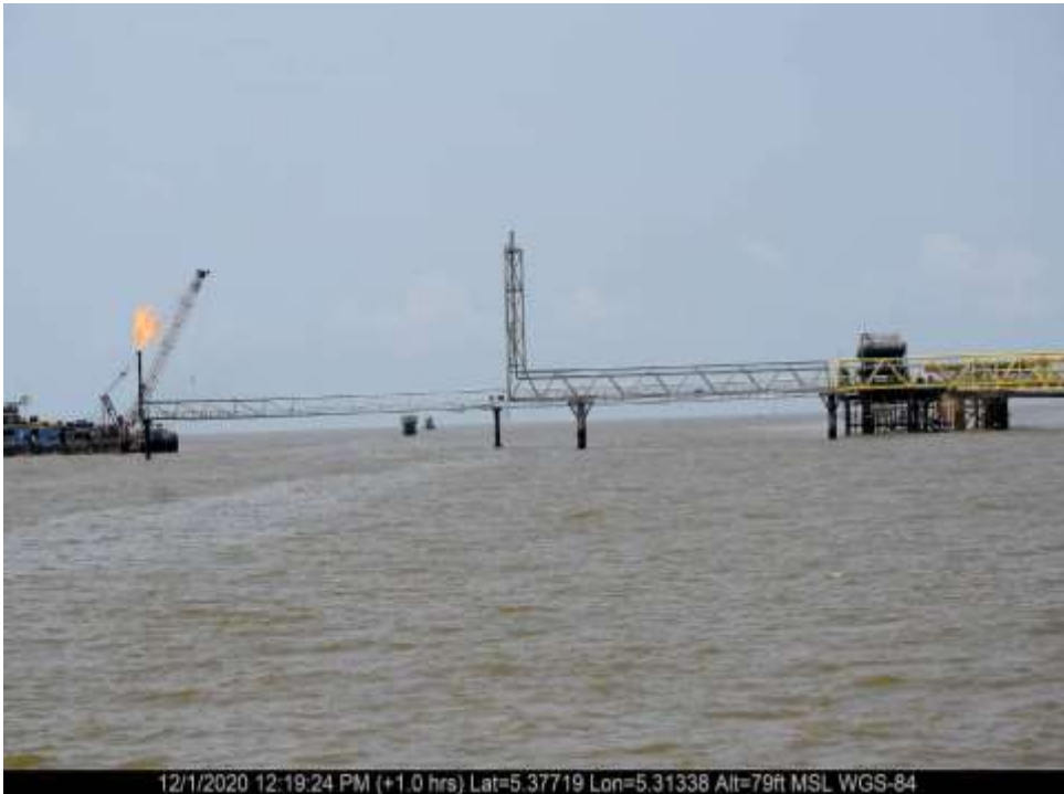
Close-up: Failed flare head on Estuary flow station flare at Ogulagha. Picture was taken during Joint Investigation of 1 st December 2020.
