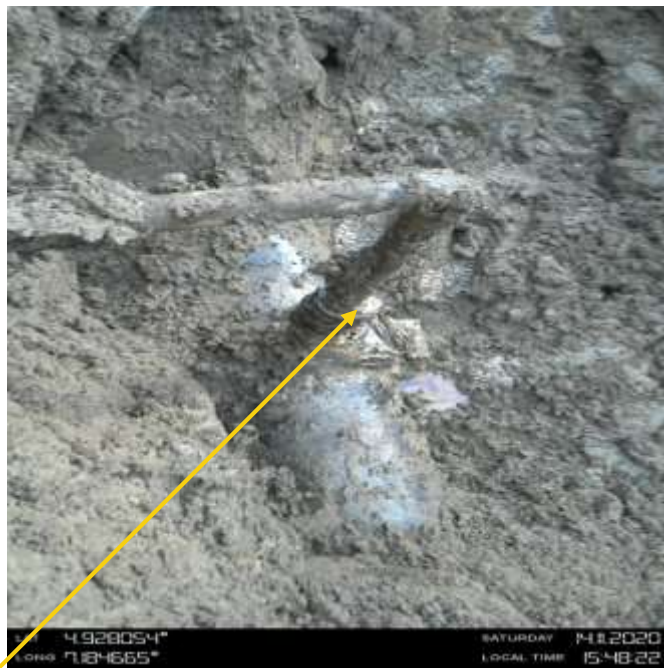
Close-up: Locally fitted clamp with 1.5inch valve installed at 12 o'clock position on 12inch Imoriver 1 - Ogale Pipeline at Okohia. Picture was taken during Joint Investigation on 14th November 2020.
