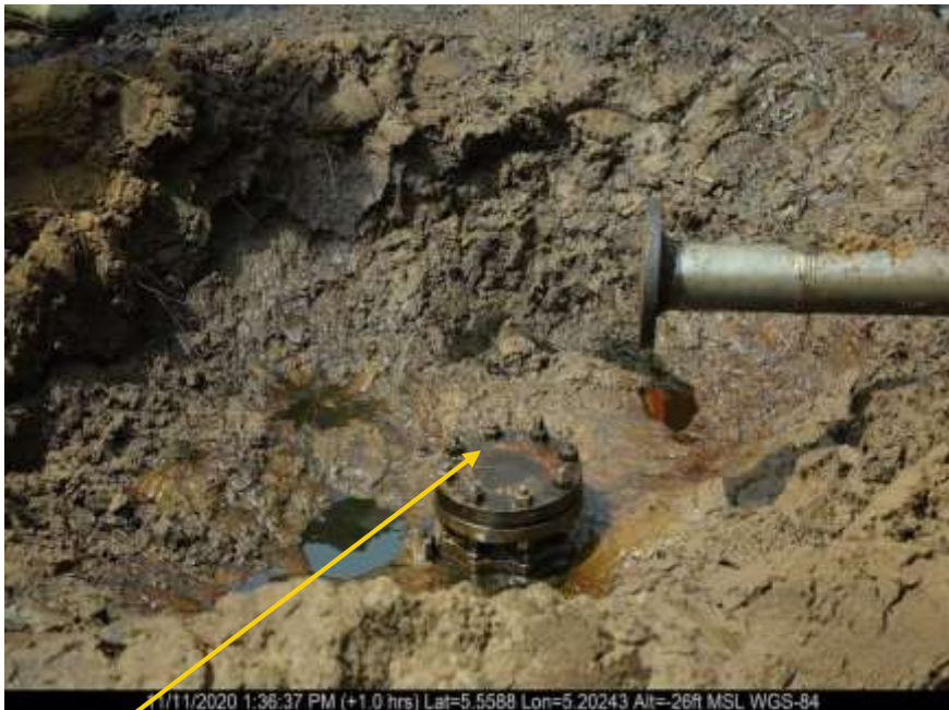
Close-up: 4inch valve with 4inch elbow reduced to 3inch pipe installed at 12 o'clock position on 20inch Trans Escravos Pipeline at Ogidigben. Picture was taken during Joint Investigation on 11th November 2020.
