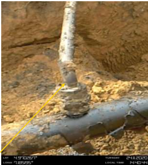
Close-up: 3inch valve connection welded on a flange at 12 o'clock position on 12inch Imo River 2 - Ogale Pipeline at Umulolo. Picture was taken during Joint Investigation on 24th November 2020
